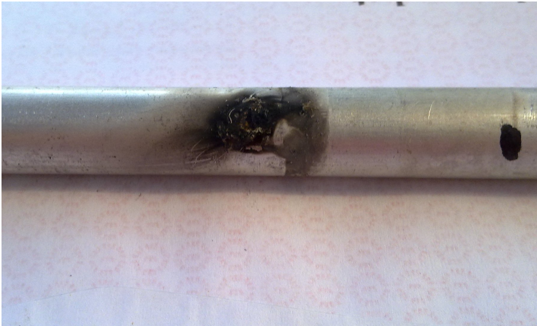
Trap pipe showing where the arcing took place.
